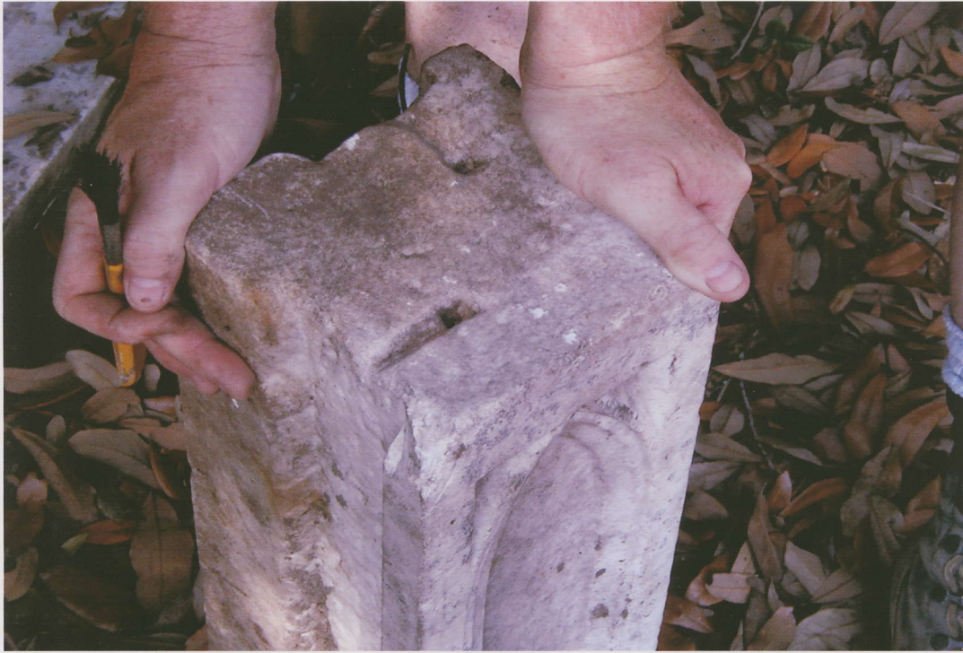
Pin holes in top of corner post.
