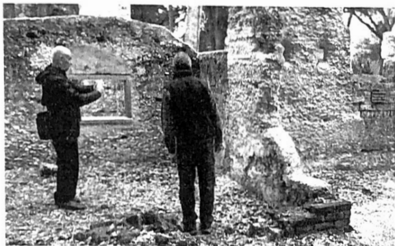
Colin Brooker snaps a picture of a crack in a tabby wall while Rick Wightman looks on.
