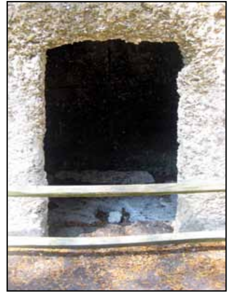
A close-up of the deteriorating door.
